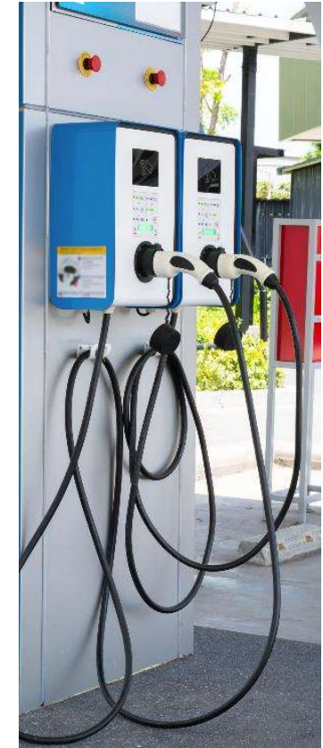
EV charging infrastructure
